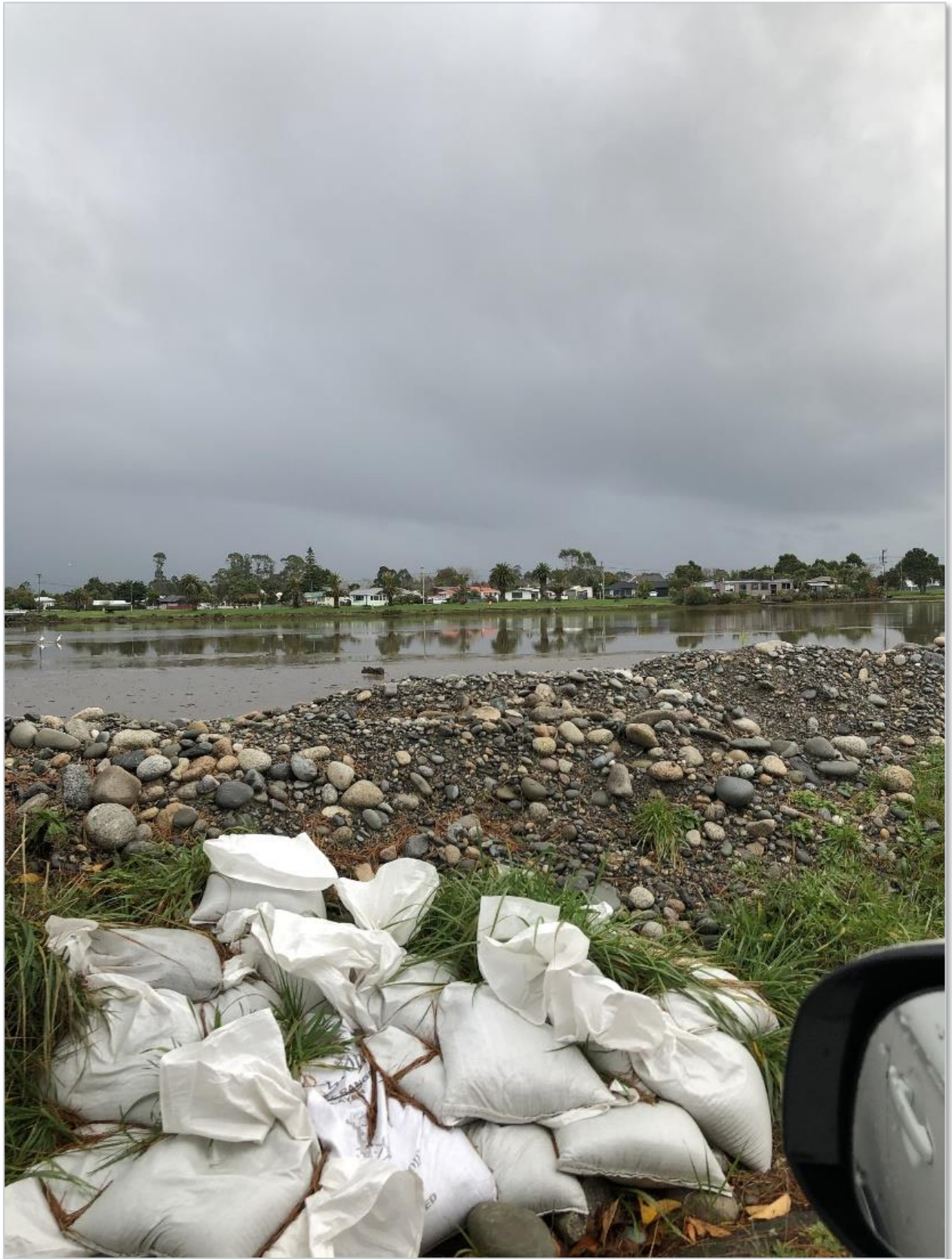
Figure 15 – Temporary stopbank at Snodgrass Road
