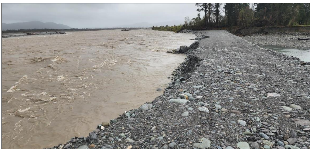
Figure 3-11: Raymond's stopbank during the 2022 July 18th/19th flood.
