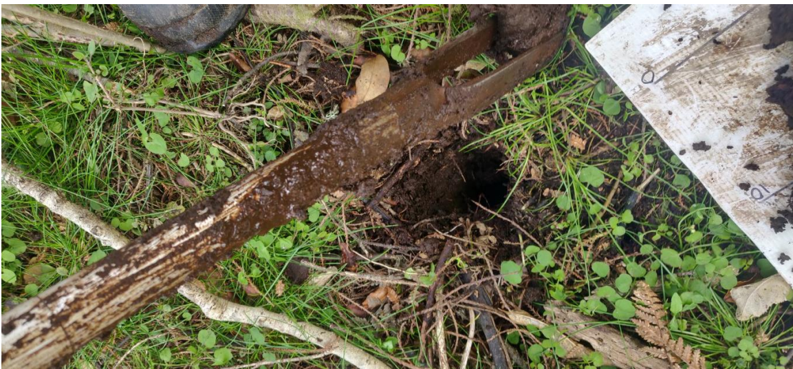
Plate 9. Evidence of a shallow groundwater table (approximately 20-30 cm below ground level) within the remnant kahikatea swamp forest within the proposed development footprint. Note the FACW wetland species Isolepis reticularis .
