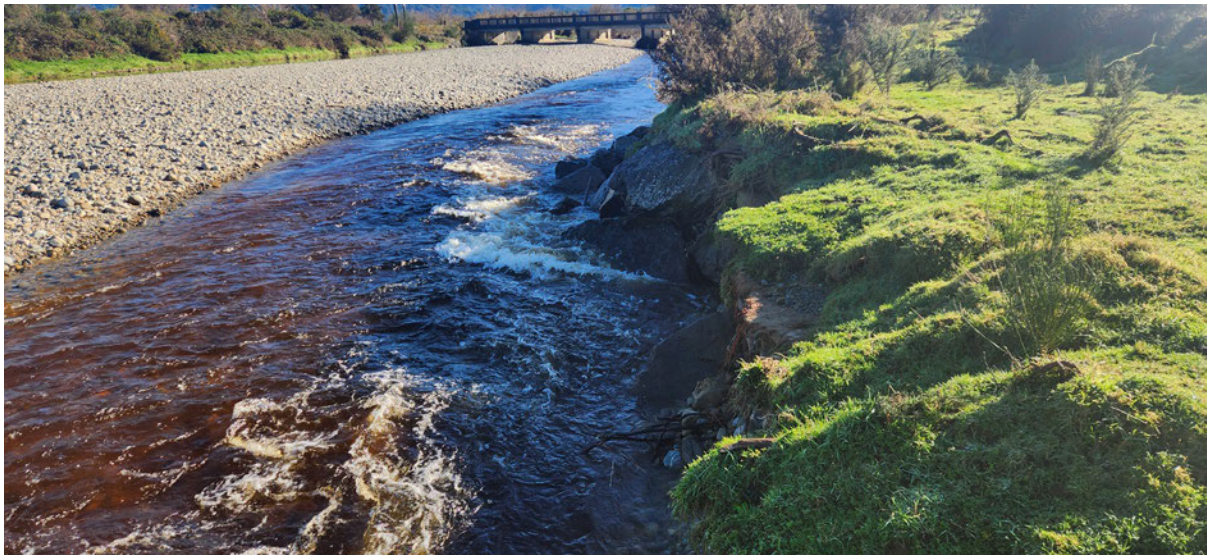
Image 1: River bank erosion July 2023
