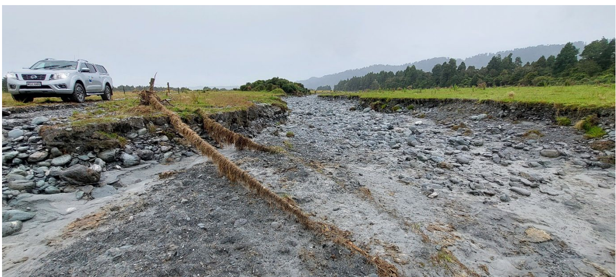
Figure 3: A new, recently formed channel through farmland resulting in scour and erosion. Fencing remnants covered in debris.
