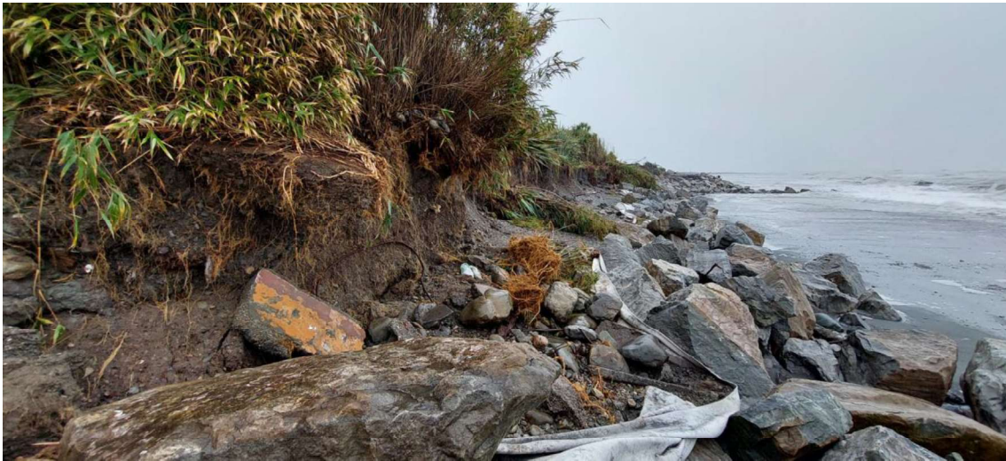
Figure 3: Coastal erosion, over-hanging vegetation, strewn filter fabric, armour rock slumping.
