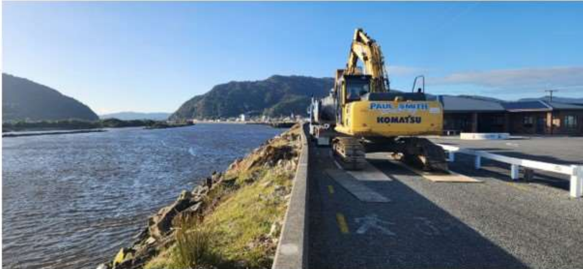
Photo 4: Picking rock off the truck deck. Rubber matting and ply for road surface protection.
