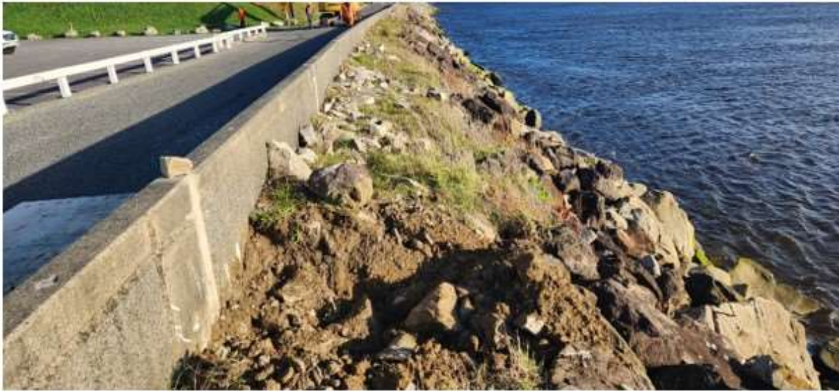
Photo 3: Partial repair showing loose material present
