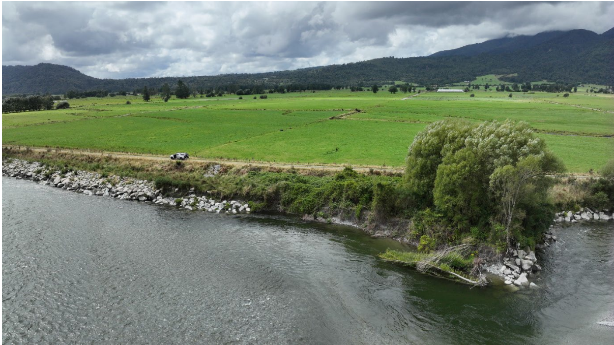
Figure 6 – View of the bank scour requiring rip-rap bank protection.
