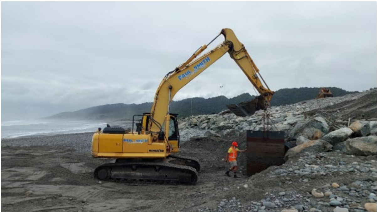
Figure 1 – The removed knife gate
