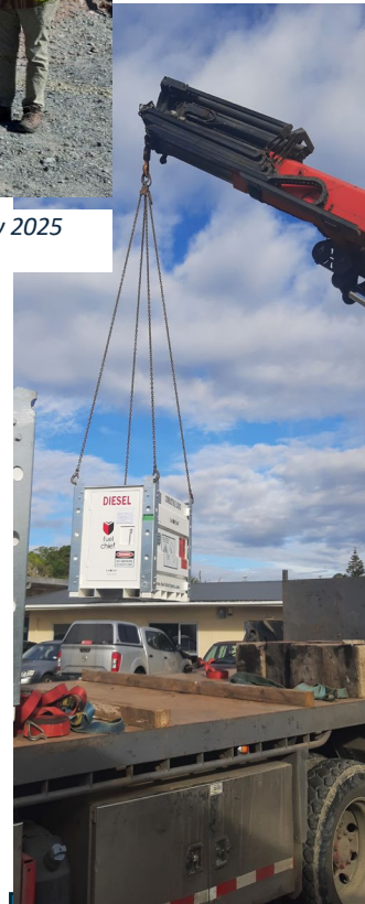
Above: The four FuelChief mobile fuel units being placed in position for West Coast Emergency Management.
