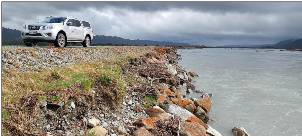
Figure 3: Slumping prior to remediation where dominant braid is directly attacking the riprap
