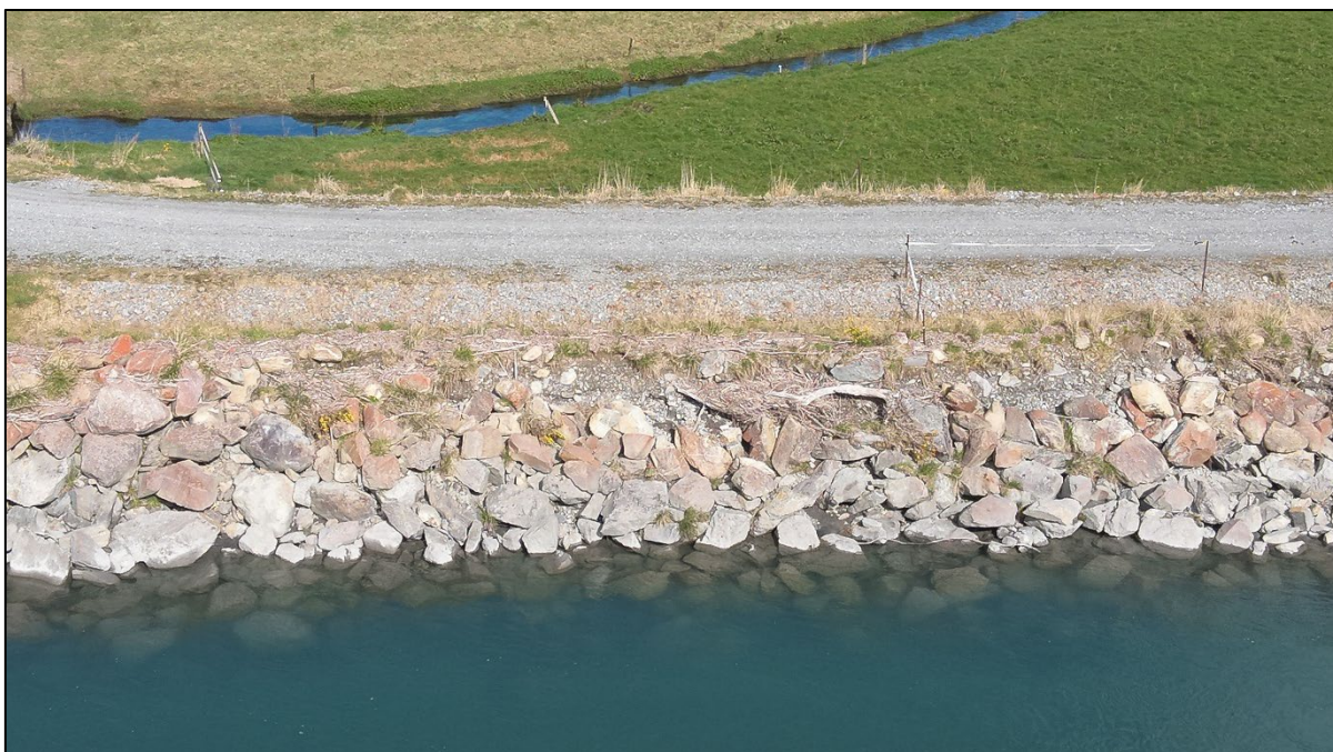
Figure 2: Example of the slumping which was present along the 75 Connect Bank
