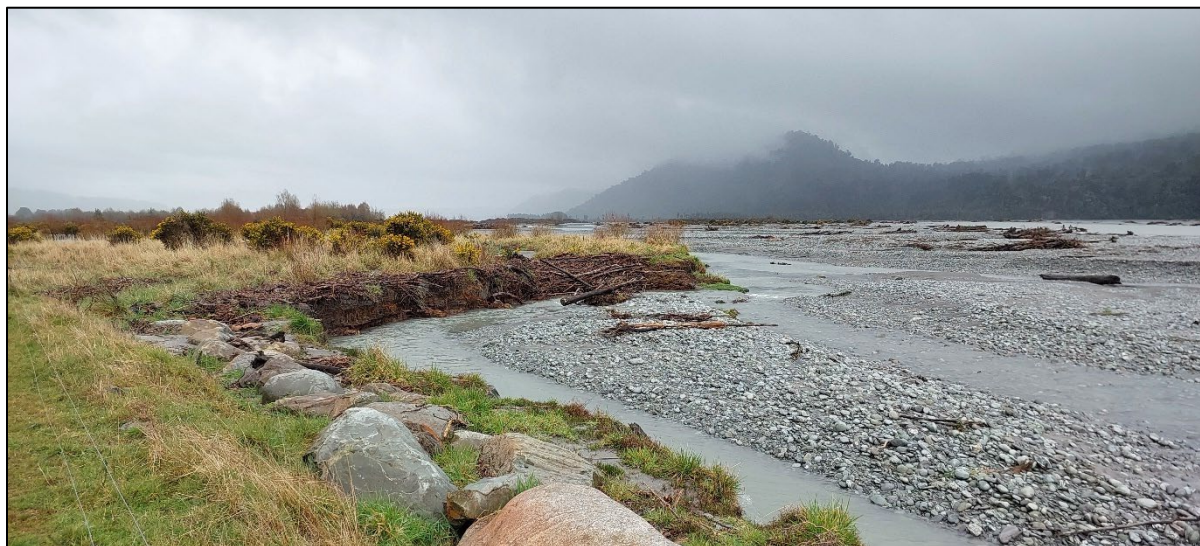
Figure 4: Riprap placed to the top of the low height stopbank, and around the bend to reduce further erosion (before repair)
