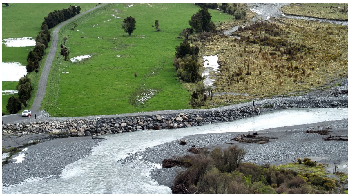
Figure 5: Tied in Retard prior to repair
