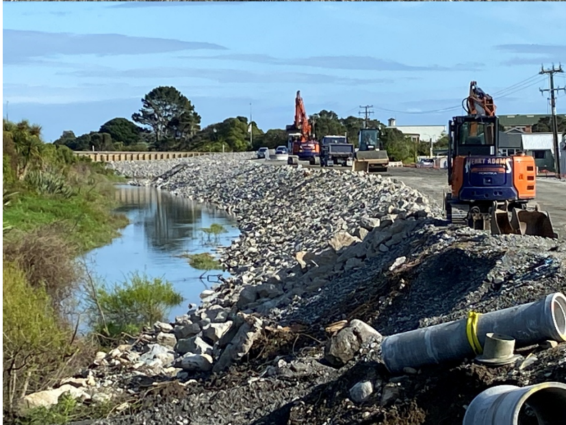
18 September 2024 Toe rock and placement of quarry rubble to Western end of bank complete, culvert extension underway.
