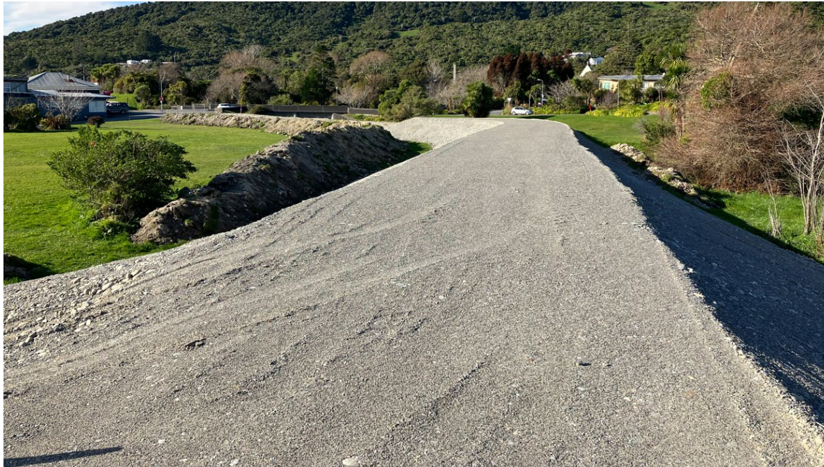
The photo to the left is from 20 June 2024, it was taken at Anzac Road looking up increasing chainage, showing the first section of bulkfill complete to finished level with final section awaiting removal of coal tar.
