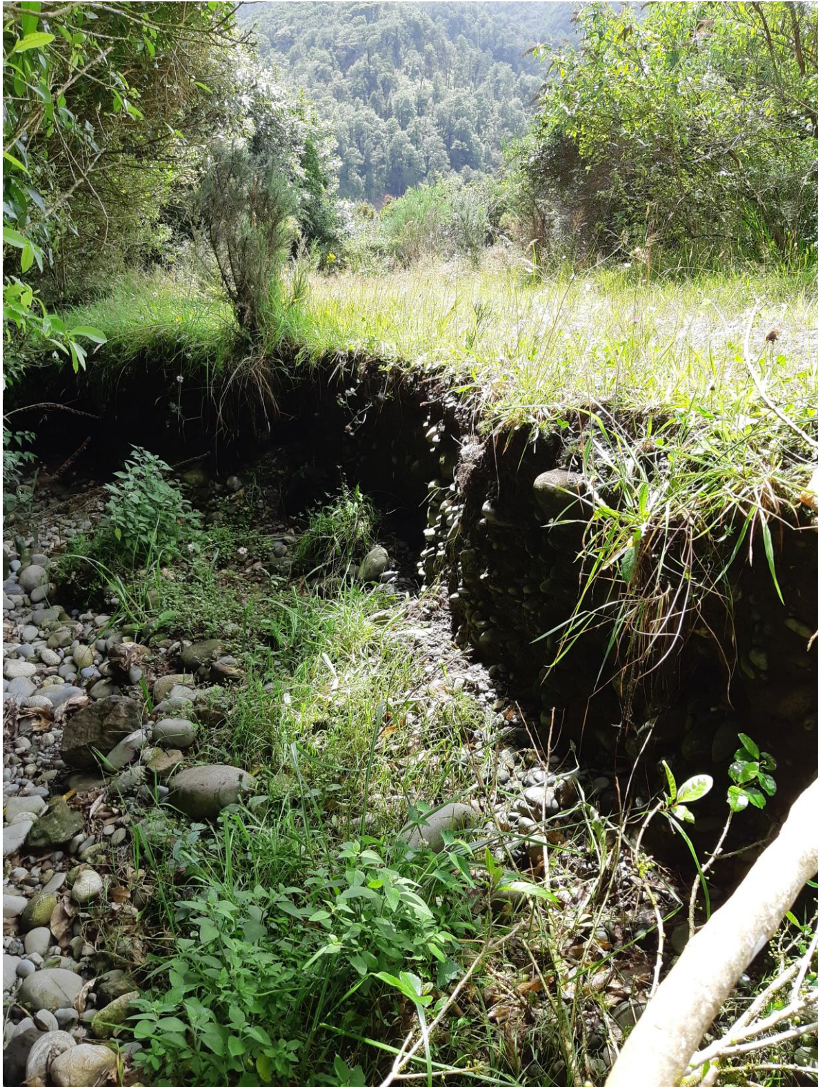
Site Photo 4 Swale drain - upslope side of access road approximately 20m below lower switchback. Recent scour of road subgrade, which is the most likely source area for recent gravel built up in stormwater channel above the KiwiRail Slip 198.7km, refer to Site Photo 2A.
