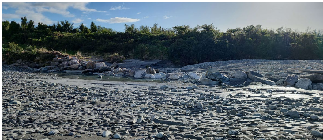
Location: Left bank, Deflector groyne, overtopping and settlement of tip of the groyne
