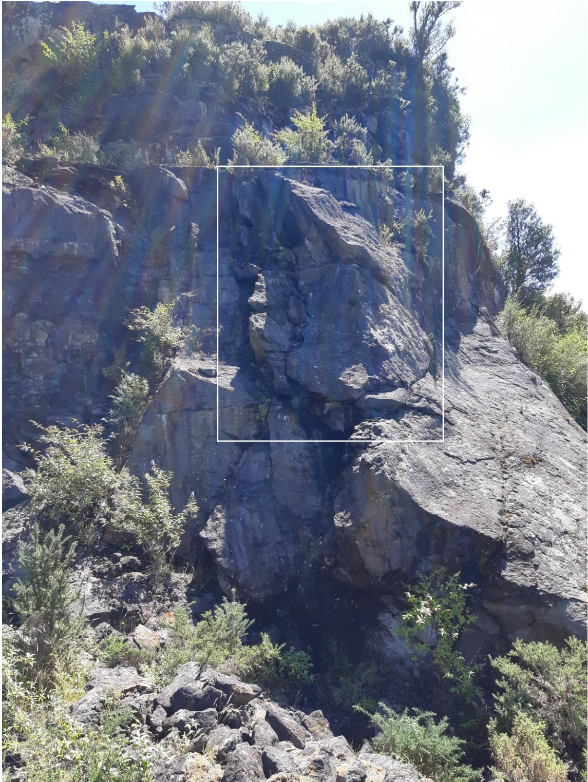
Site Photo 12 Lower batter of the Nose. A large slab (estimated at 3x2x1m) of rock appears to be partly detached.
