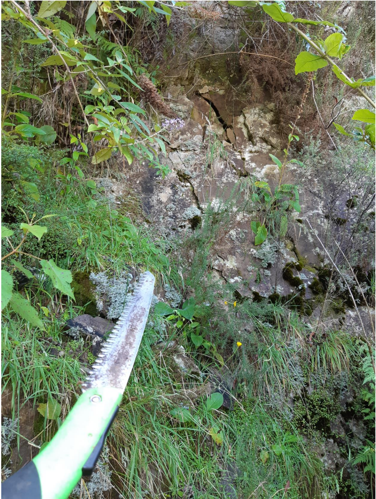
Site Photo 8 Developing surface cracks observed in rockface on southeastern side of the Pinnacle.
