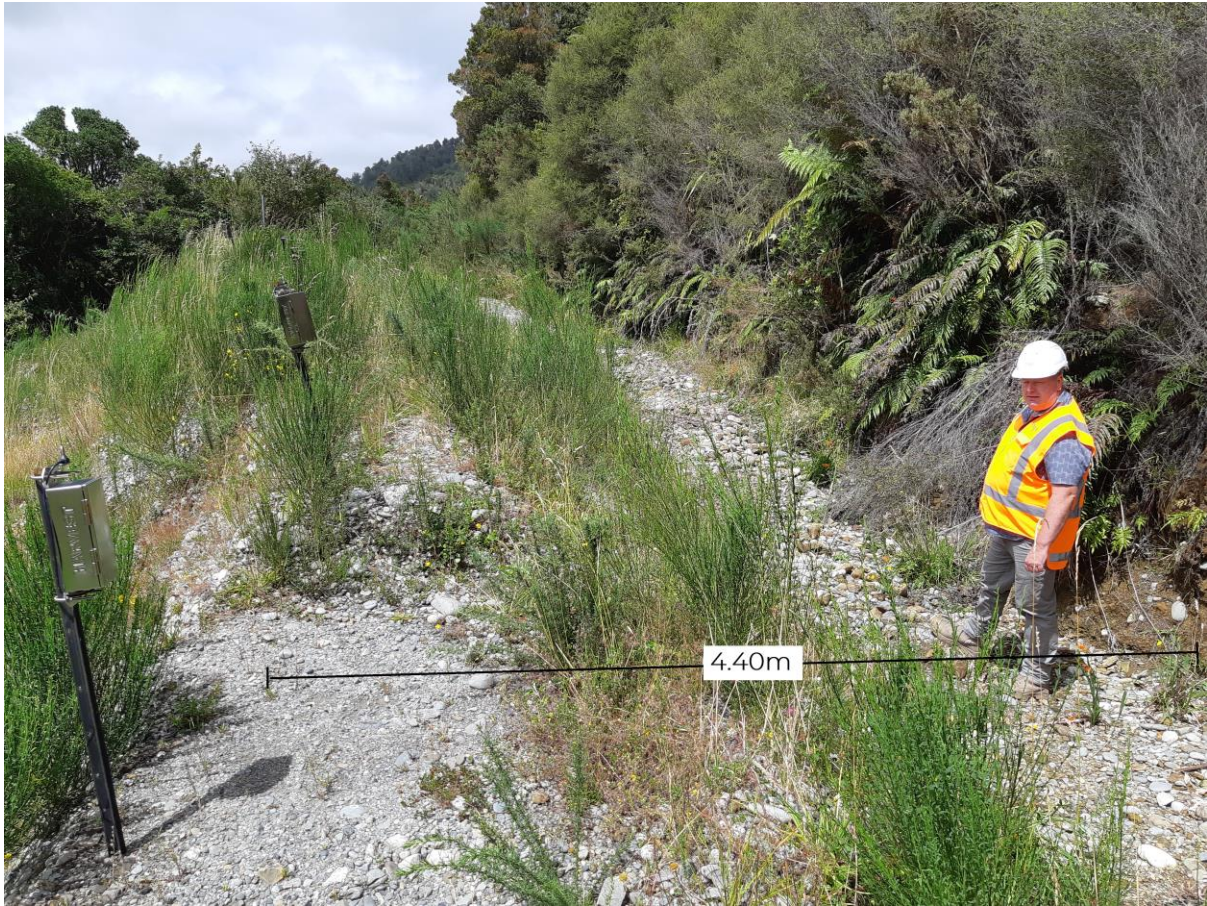
Site Photo 1 Failed section (KiwiRail Slip 198.7km) of the lower part of access road to Kiwi Quarry. KiwiRail has installed a series of tiltmeters along a bund straddling the crest of the slip to monitor the slope. The road width is currently 4.40m at the narrowest point.
