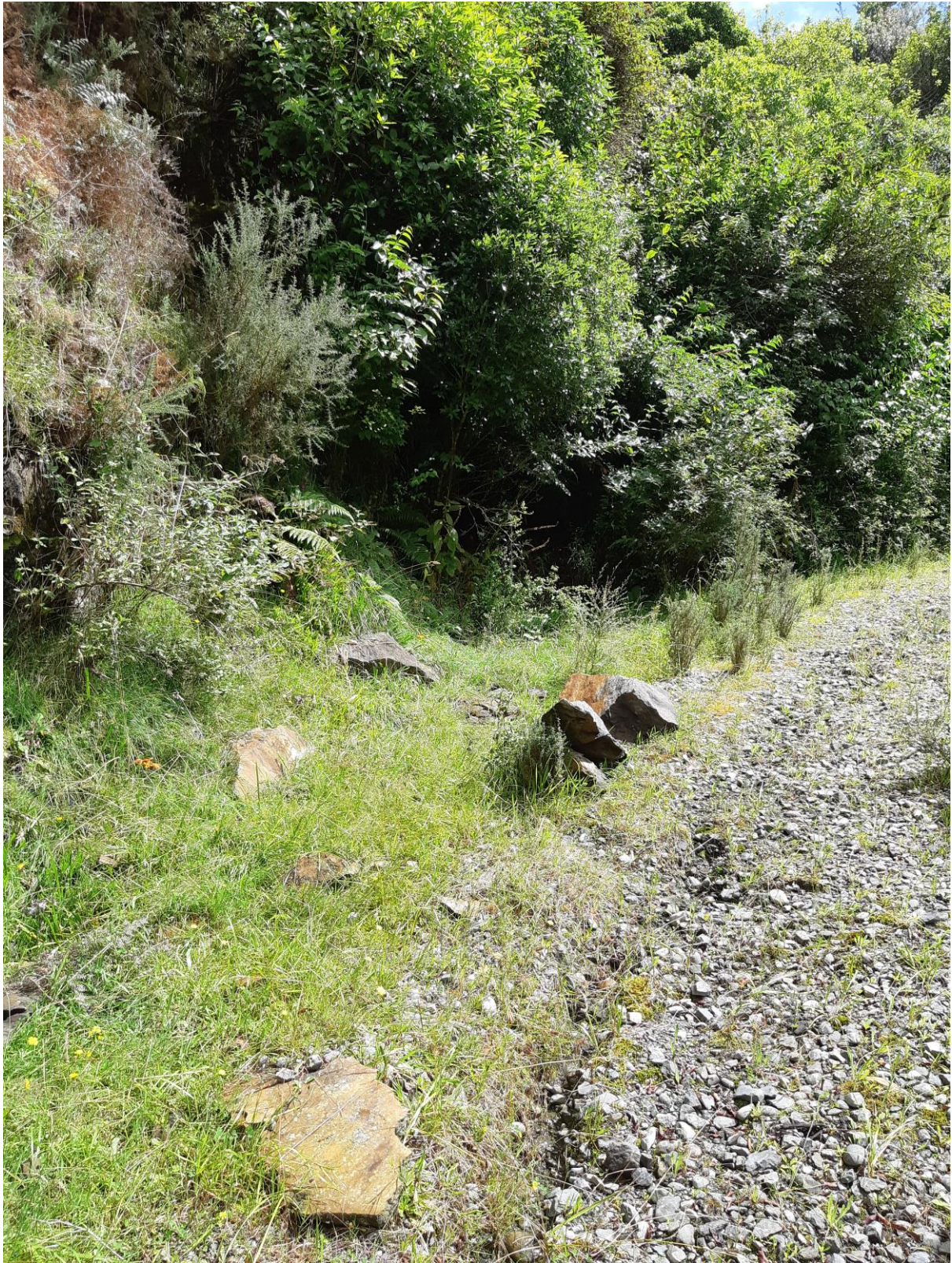
Site Photo 5 Rockfall in shoulder of access road by lower switchback. Block size up to 0.80x0.55x0.45m maximum size.
