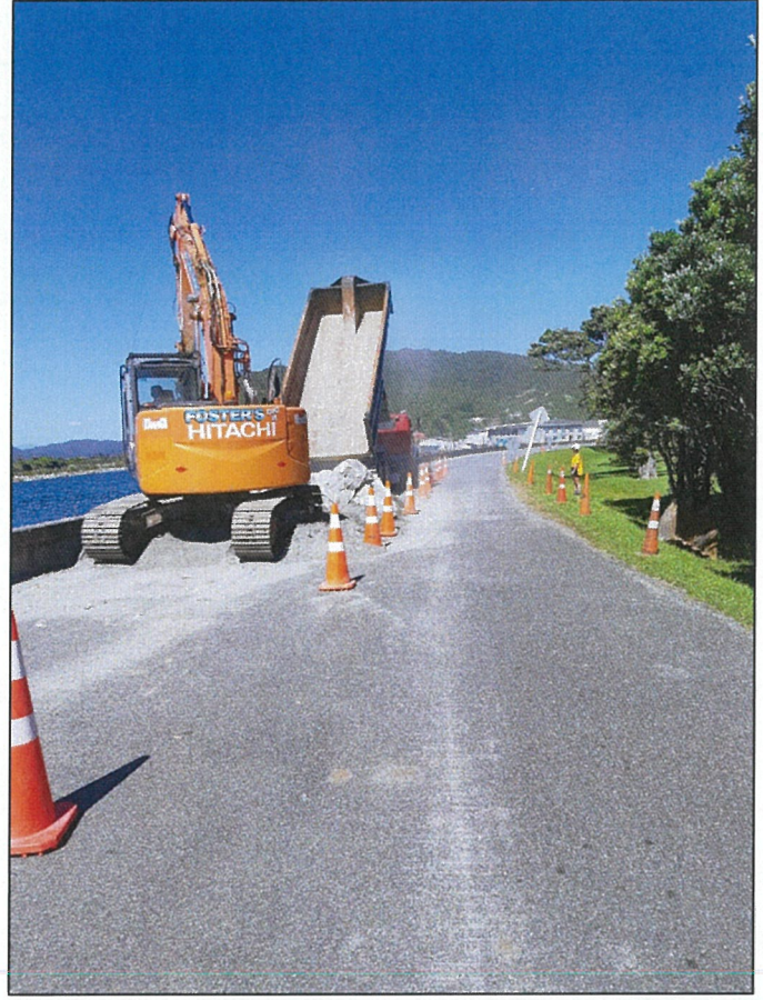
Unloading rock. Spotter used for traffic due to the narrow width of the road.
