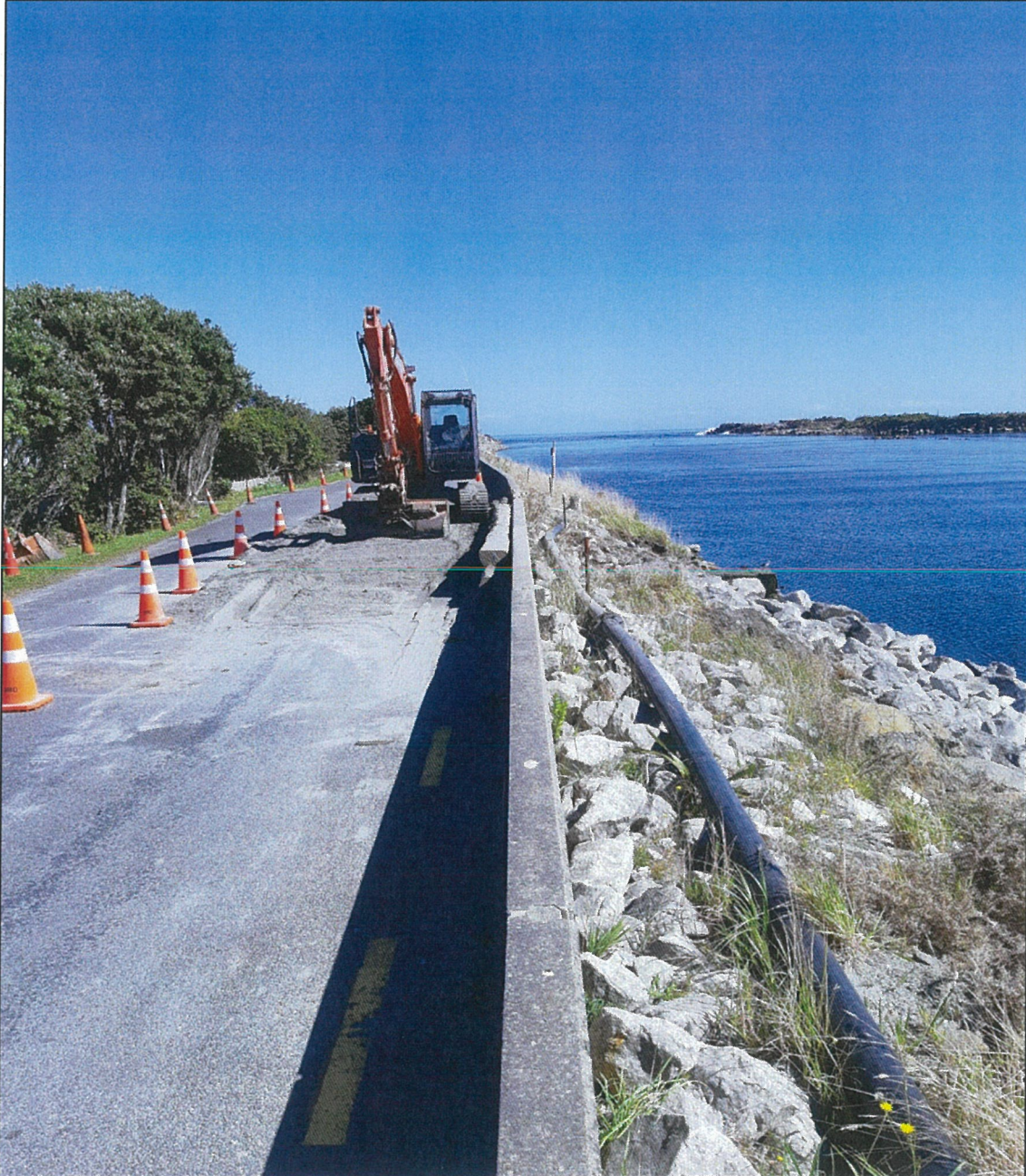
Zero-swing digger, showing the crusher dust base used to protect the road surface and the concrete floodwall.
