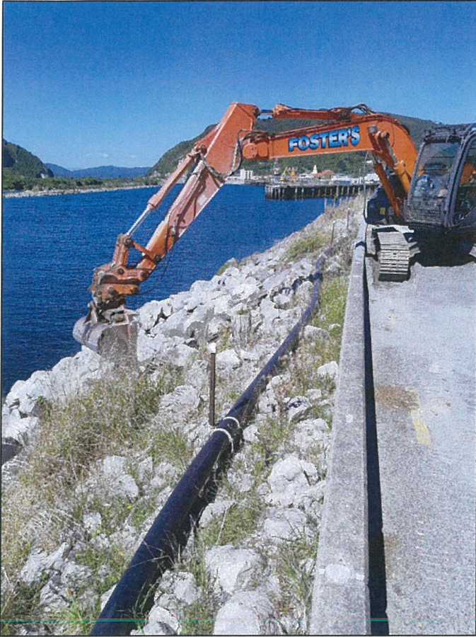
Zero-swing digger, showing the crusher dust base used to protect the road surface and the concrete floodwall.
