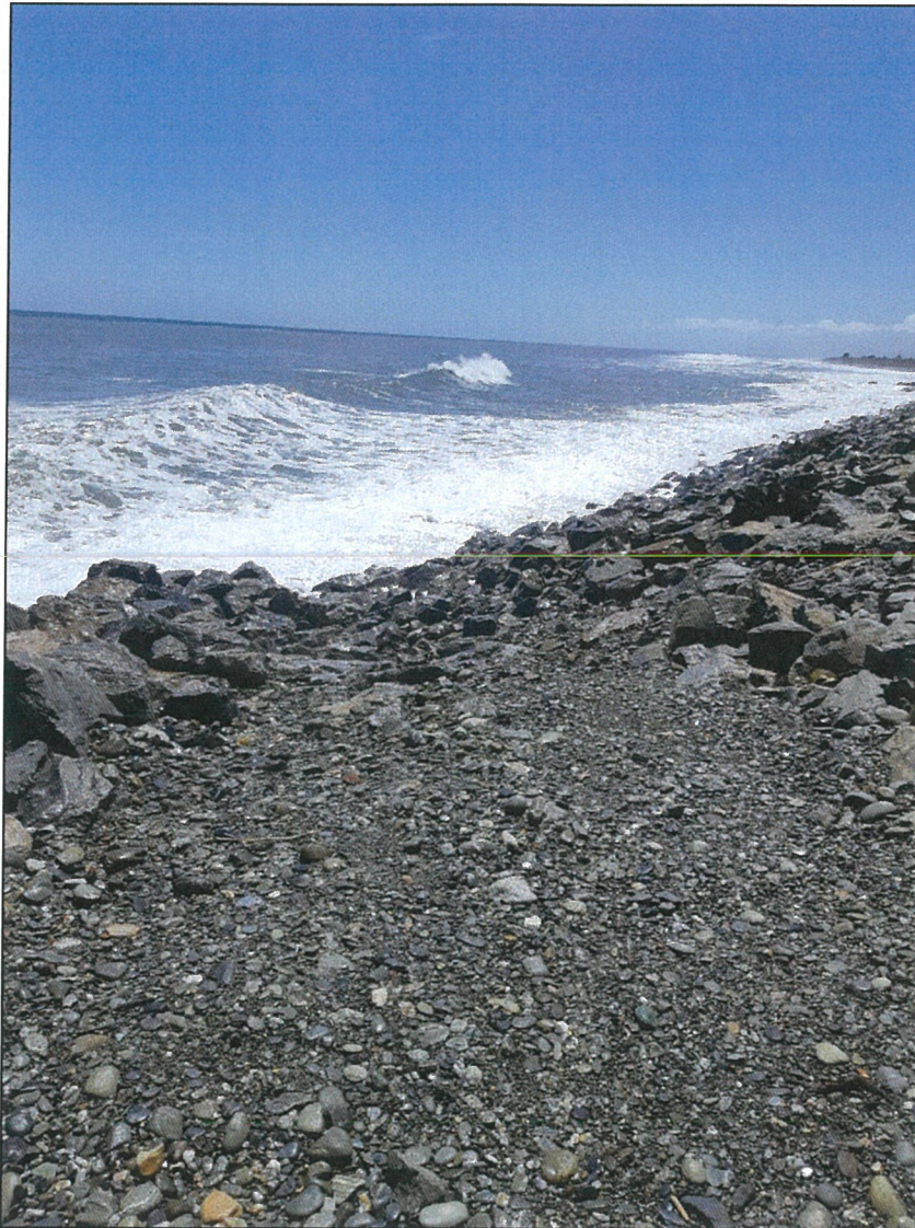
Damaged Pedestrian Access Ramp
