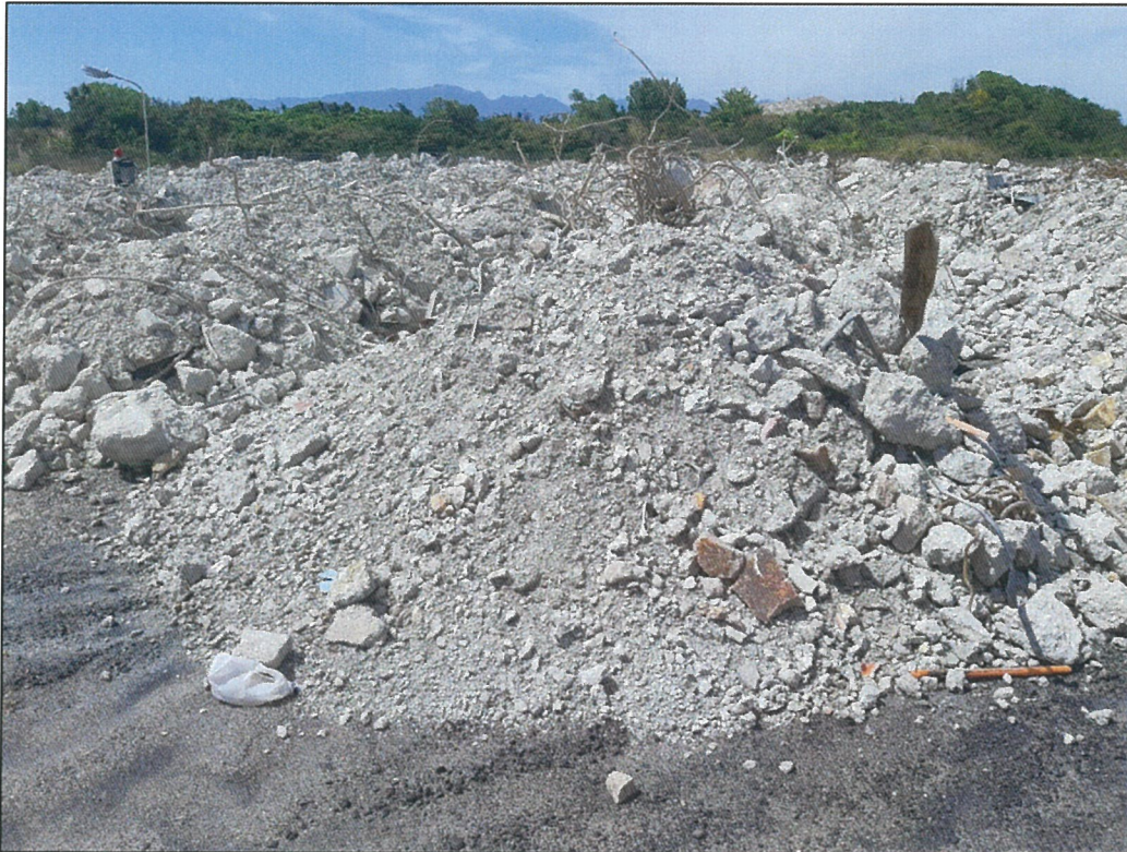
Concrete that has already been broken up by an excavator, but still has reinforcing steel
